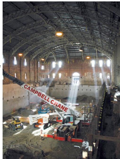
GBD Architects was able to adapt an historic armory for use as a theater by building the new structure inside the old one. Christopher Smith/courtesy Portland Historic Rehabilitation Fund
